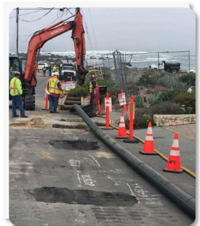
Needed Road Maintenance
