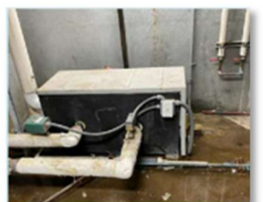
Golf Restaurant HVAC
